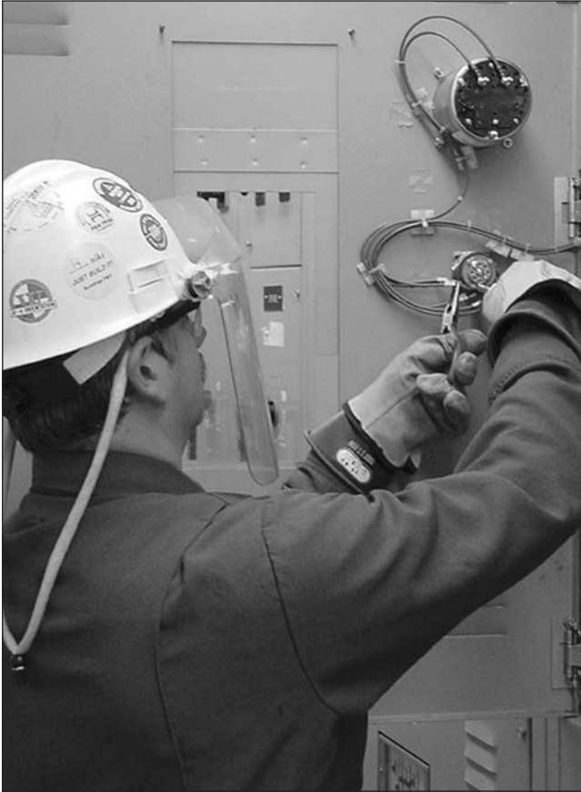
A workman with suitable personal protective equipment (PPE) working on energized equipment.
